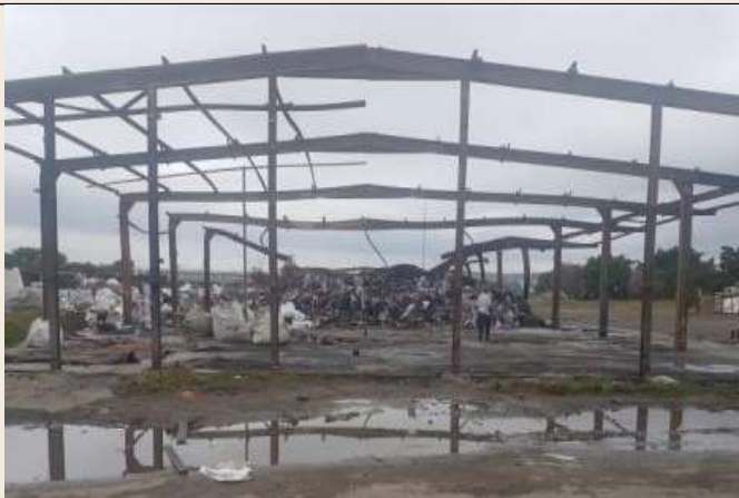
A: Burnt overhead structure
